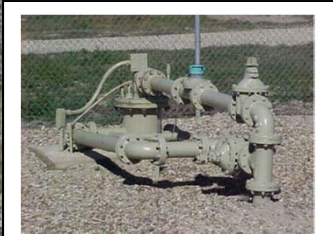
Shallow Groundwater Dewatering Pump
